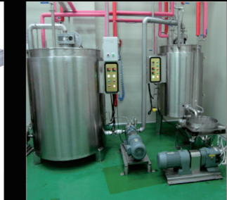
巧克力保温缸 Chocolate storage tank
